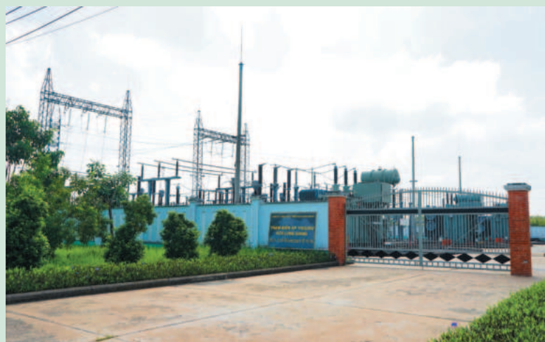
The power infrastructure of Long Jiang Industrial Park is developed to effectively support the business requirements of investors
